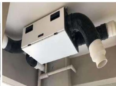
Fresh air system
